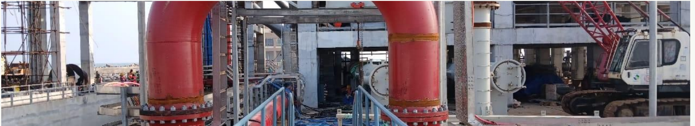
Fire-line pipe rack and walkway, completed run.
