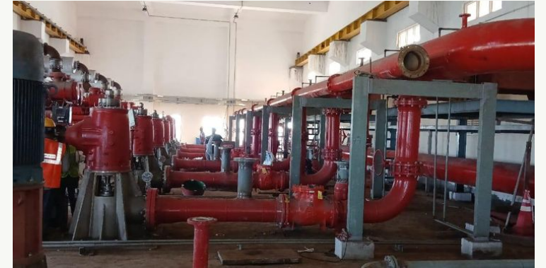
Fire pump house piping
